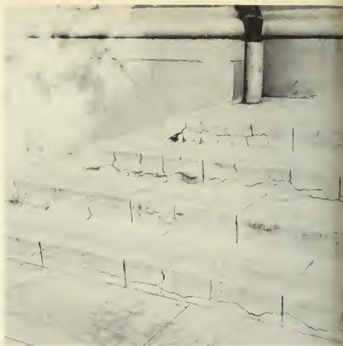
FIGURE 10. Cracking in steps, Law Building, University of Southern California, Los Angeles.
